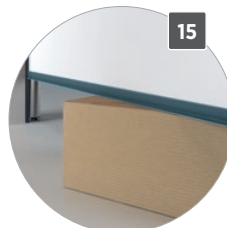
15 Overload safety device In automatic doors; the door leaf stops and reverses when the bottom edge contacts an obstacle.
